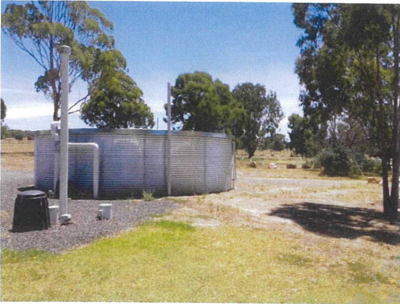
Figure 4 Winton Wetlands Wastewater Treatment System
